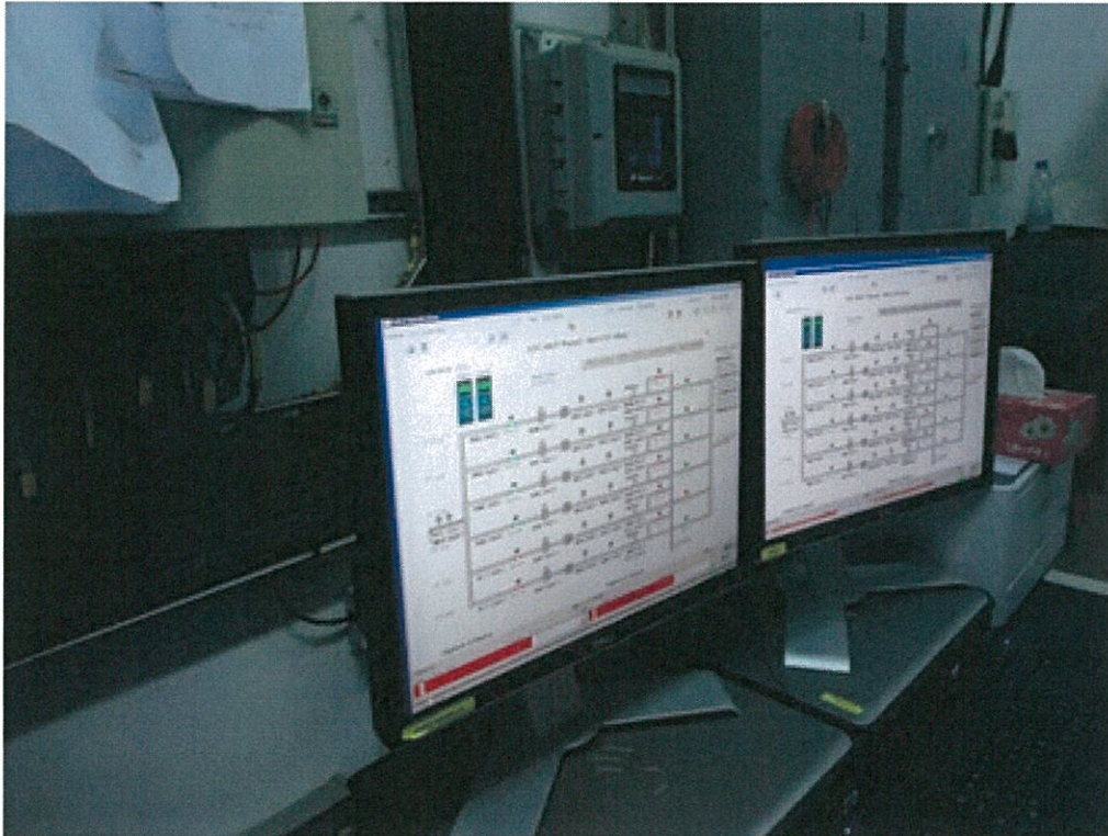
Platform B Metering Station HMI
