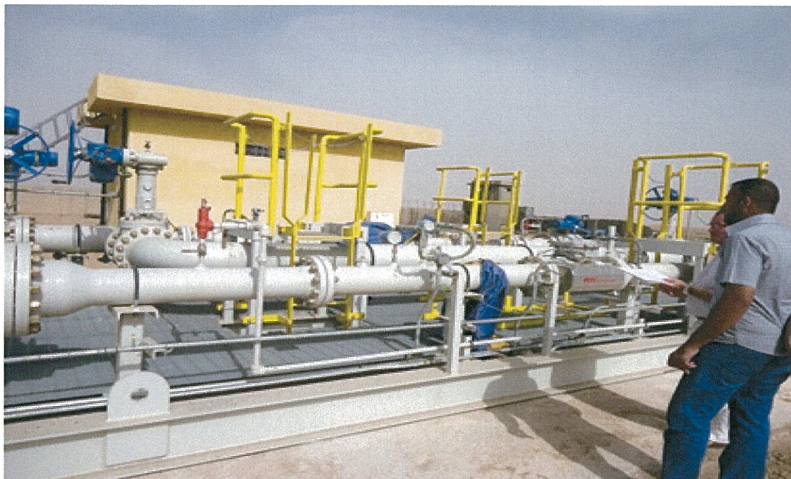
New Missan Refinery Inlet Metering Skid
