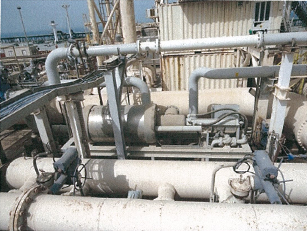
Platform B Metering Station Compact Prover and Master Meter
