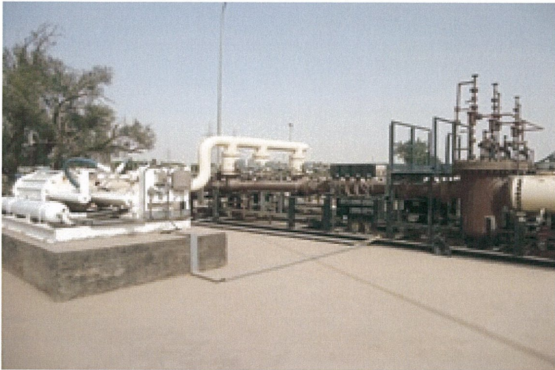
Al Zubair 3 stream and compact prover metering skid
