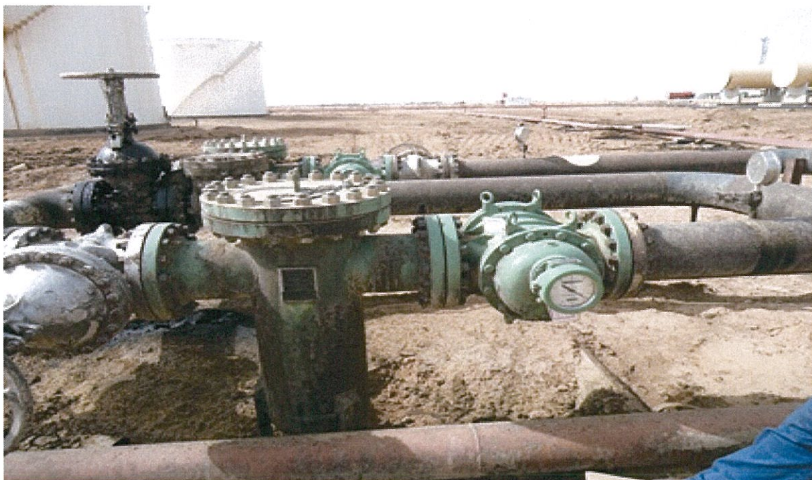
Missan Refinery Inlet Meters
