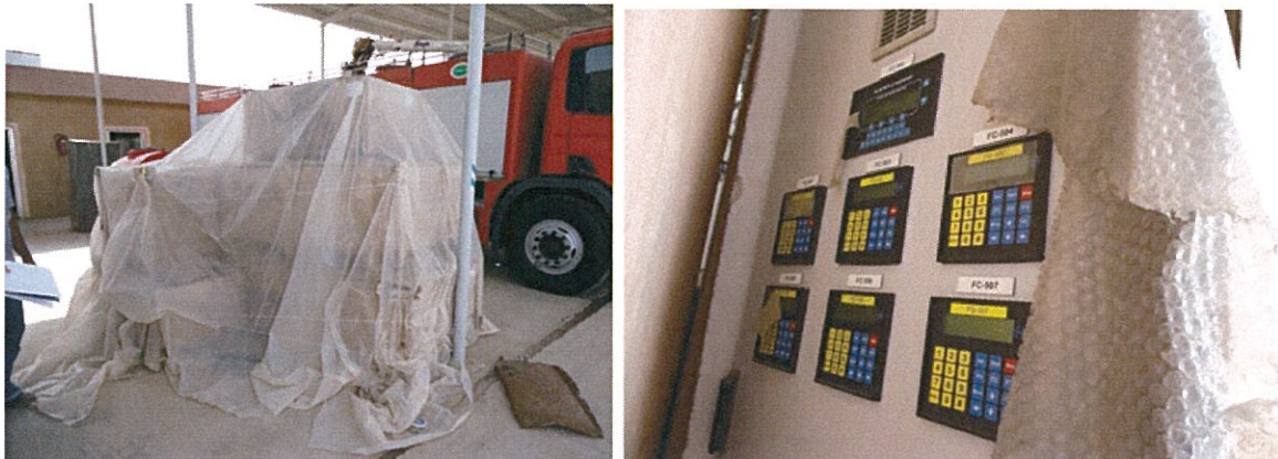
New Corilos Meters and Panel
