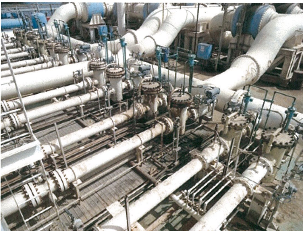
Al Basrah Oil Terminal Platform B Metering Station
