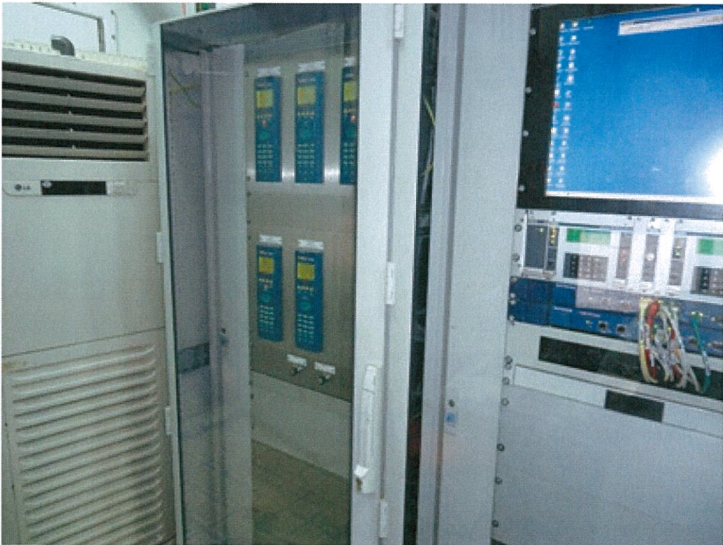
Platform B Metering Station Stream Computers
