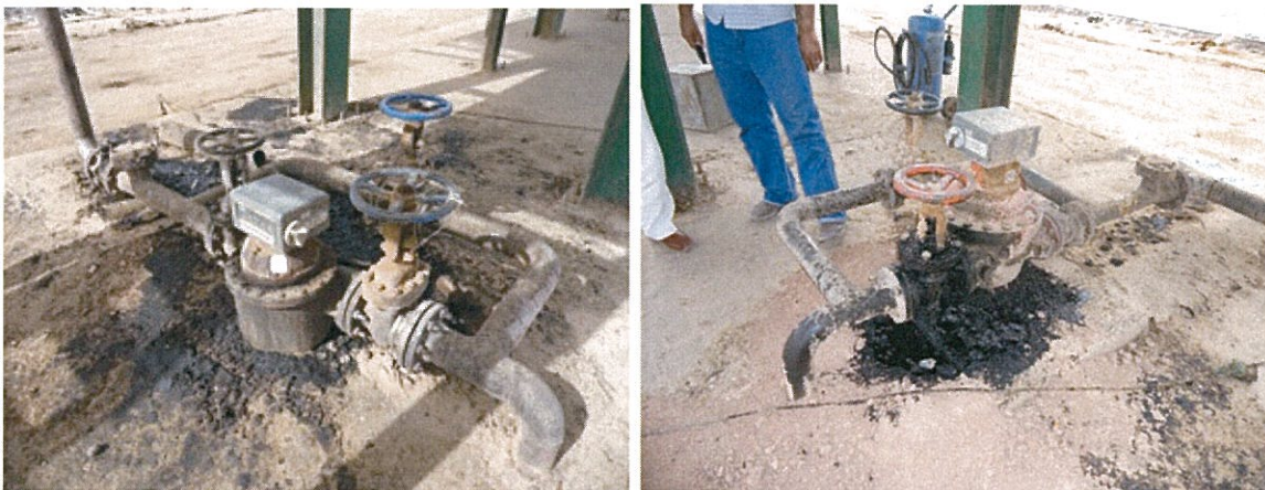
Heavy Fuel Oil meters FQ24-1 & 2
